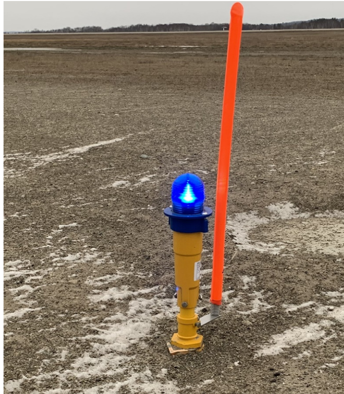
Figure 35 - Taxiway Edge Light Alpha and Bravo
