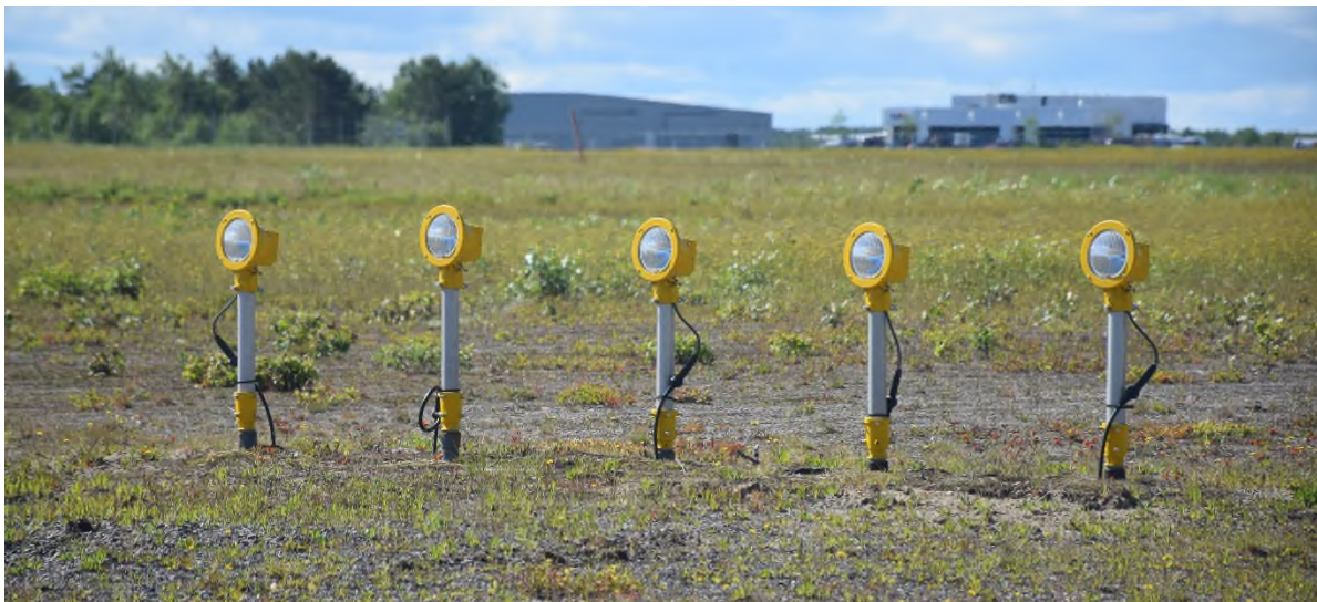
Figure 478 - Short Simplified Approach Lighting with Runway Alignment Indicator Lights (SSALR) Row of White Lights
