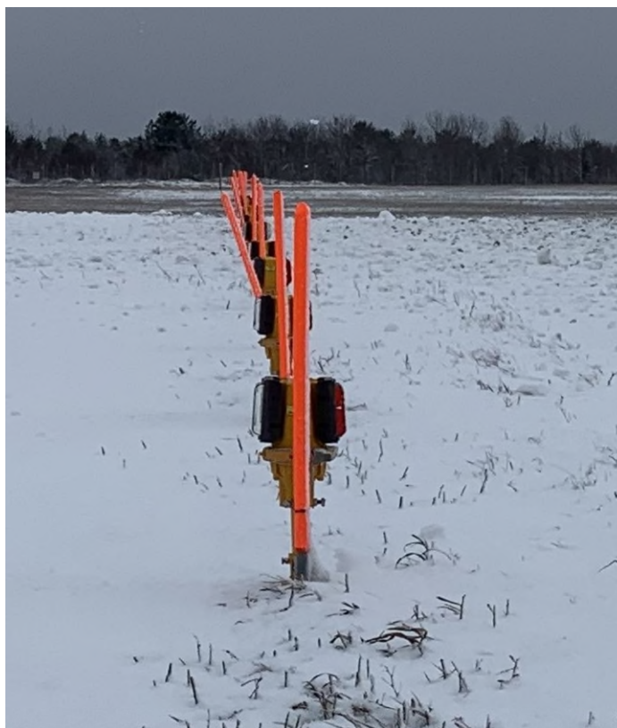
Figure 30 - Runway End and Threshold Lights on Runway 22
