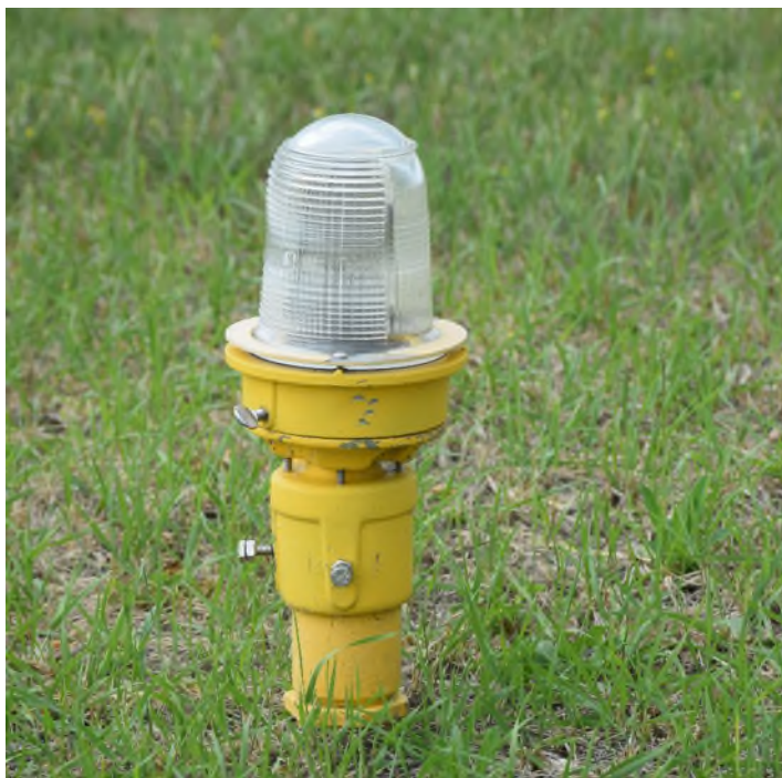
Figure 23 - Runway Edge Light located on Runway 12-30
