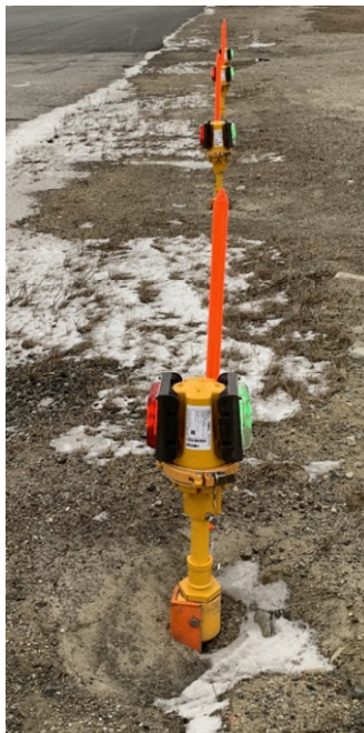
Figure 27- Runways End and Threshold Lights on Runway 04
