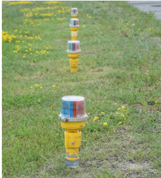
Figure 26 - Runway End and Threshold Lights on Runway 12 and 30
